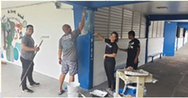
From 2010-2018, DMA adopted and helped prepare Merizo Elementary School for the start of the school year. Employees of DMA and Guam National Guard assisted in painting, water blasting, pruning of plants and trees, fixing electrical and plumbing at no cost to the school.
