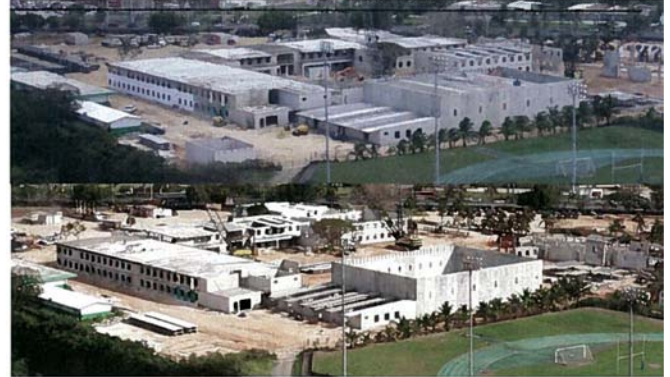
Feb 12, 2011 Precast Erection Phases 2, 3 & 4; Gym Walls erected, Precast Production Ongoing, U/G Utilities Ongoing
