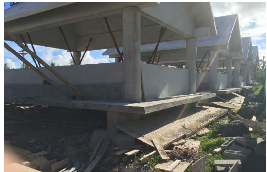
Image 4. Photo of hut construction at Flood Zone VE taken on March 22, 2016 by DCA President.
